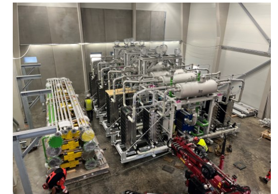
1 st electrolyzer (out of 3)
