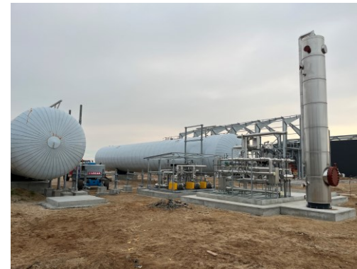
CO 2 -storage tanks
