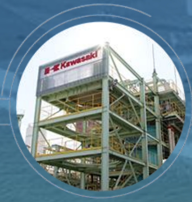
H2-Production and Liquefaction
